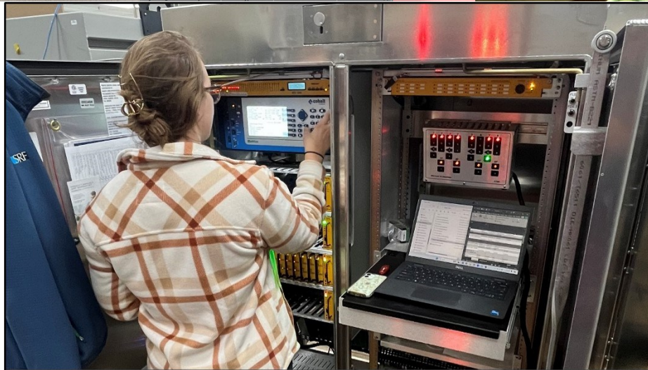
Stage 4 Testing, Cabinet Testing at MnDOT's ESS Office. Source: SRF
