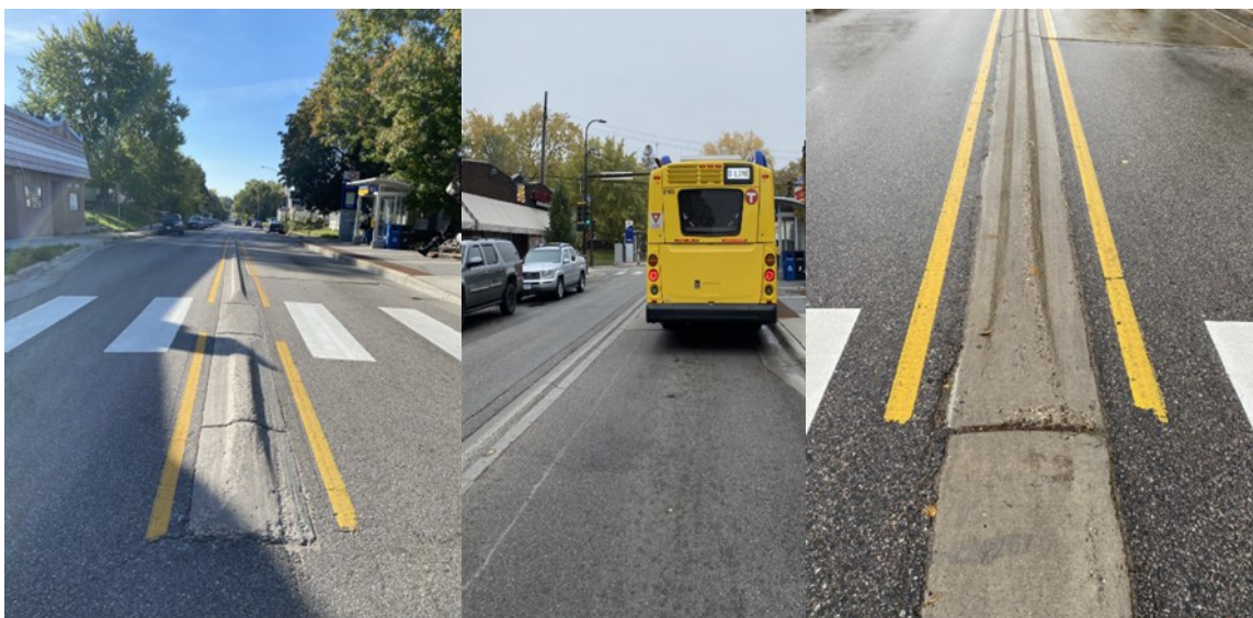
Figure 1: Example images of a hardened centerline on the D Line BRT corridor
