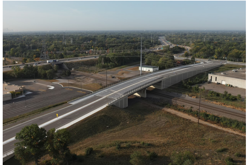
The new configuration is a four-lane urban roadway curb with gutter, storm sewer, a sidewalk on the north side, a trail on the south side, and center left turn lanes.
