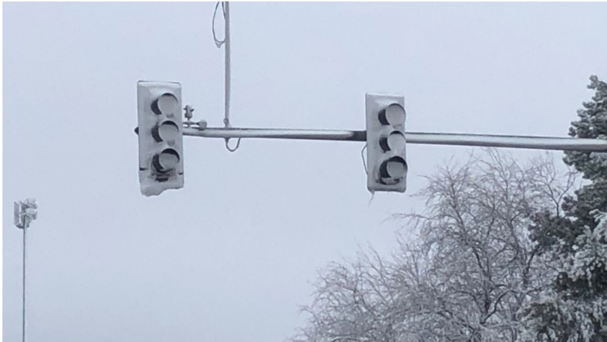
Snow Covered LED Signals. Source:
