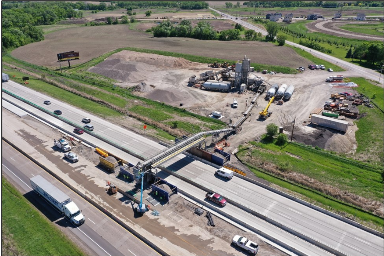
Concrete conveyor used on the I-94 Design-Build Project, Rogers to Maple Grove, MN (Source: C.S. McCrossan)
